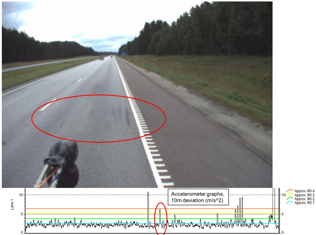
Figure 63_4. Bump on road surface (related to frost?) in lane 1, at chainage 43 700m.
