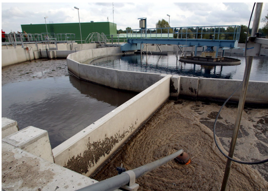
Modern sewage treatment plant in Kõsti in Viljandi was opened two years ago.
