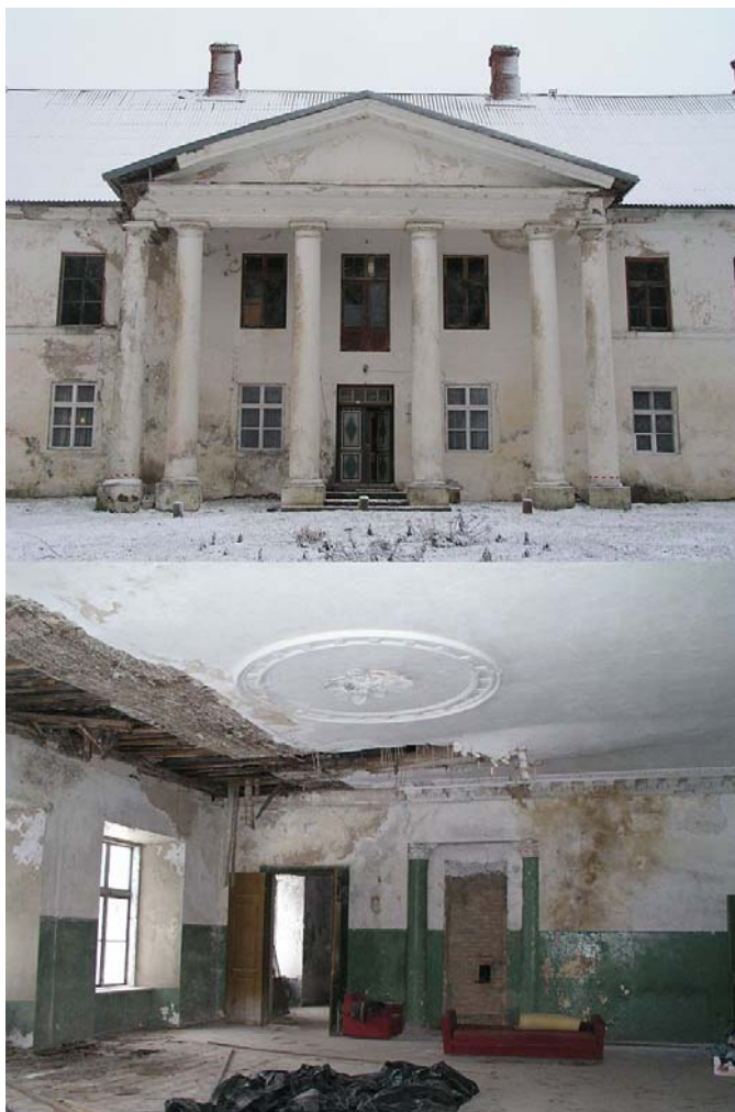
Architectural monument in a very poor condition – main building of Kirna manor in Järva County, private property.
